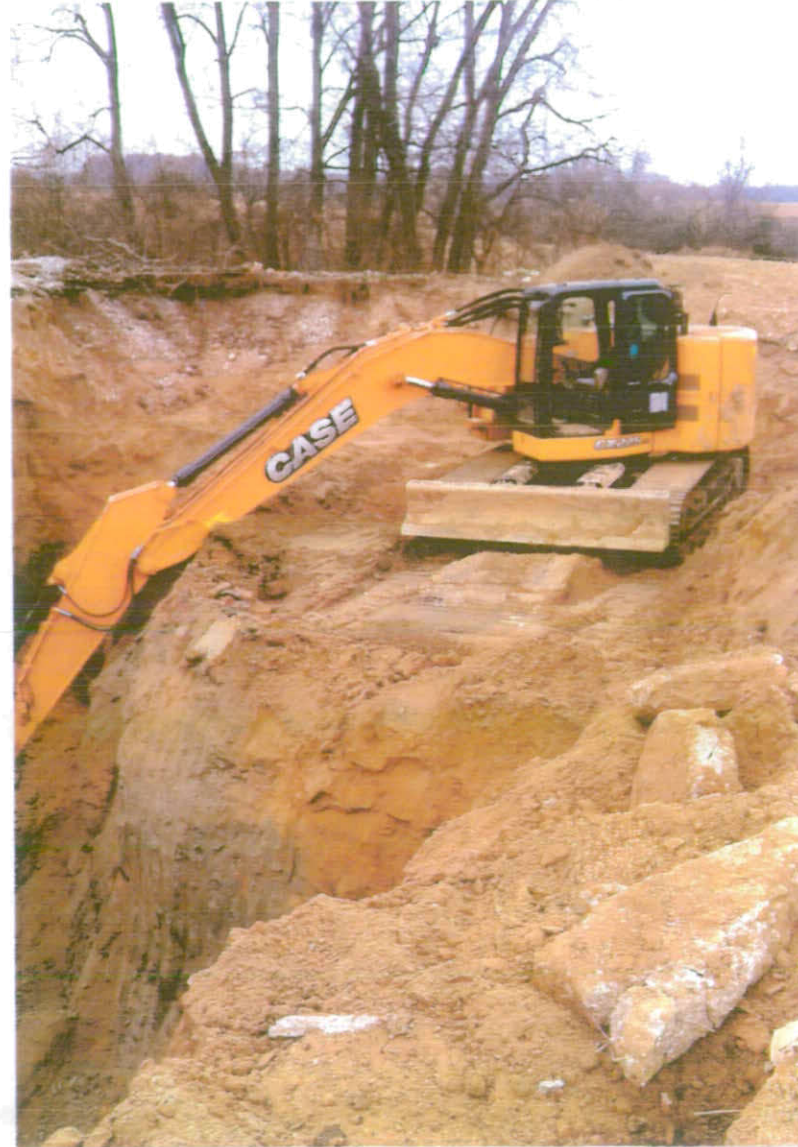
12/04/2013: View of Excavation looking from the East wall toward the Northwest corner of the Excavation
