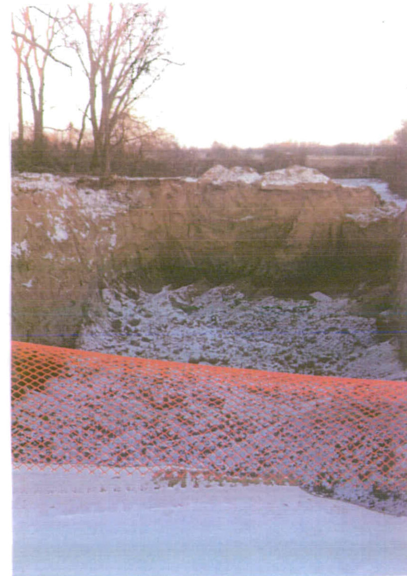
12/10/2013: View of Excavation looking from the South wall toward the North wall of the Excavation
