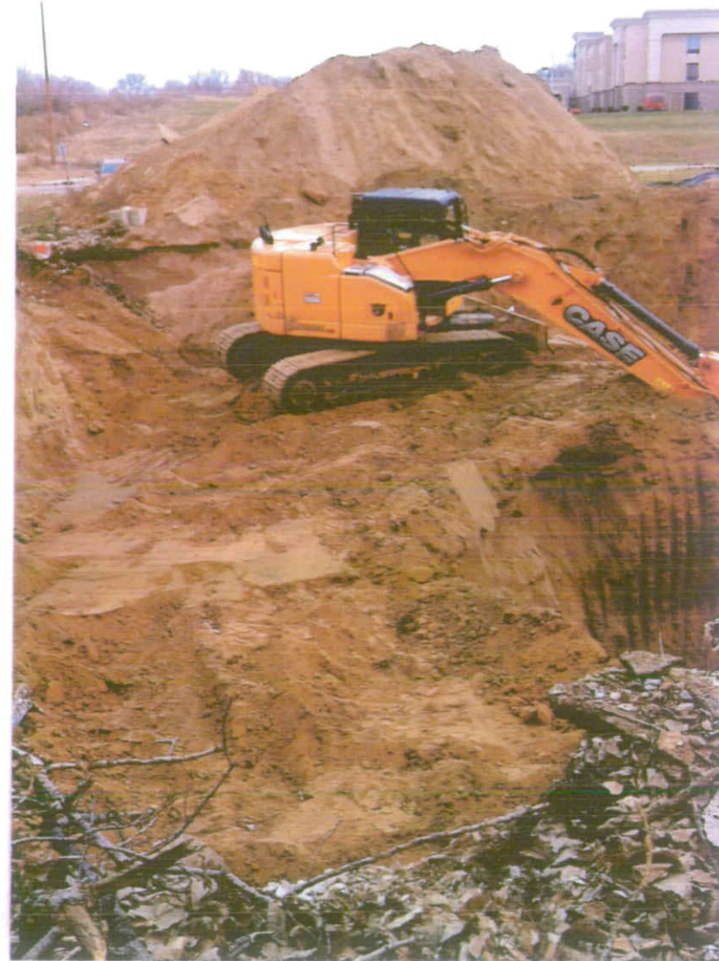
12/04/2013: View of Excavation looking from the West wall toward the East wall of the Excavation
