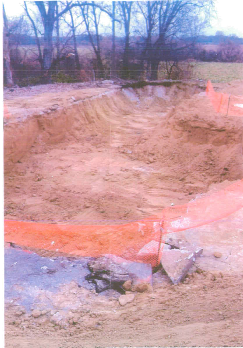
11/20/2013: View of Excavation looking from the South wall toward the North wall of the Excavation
