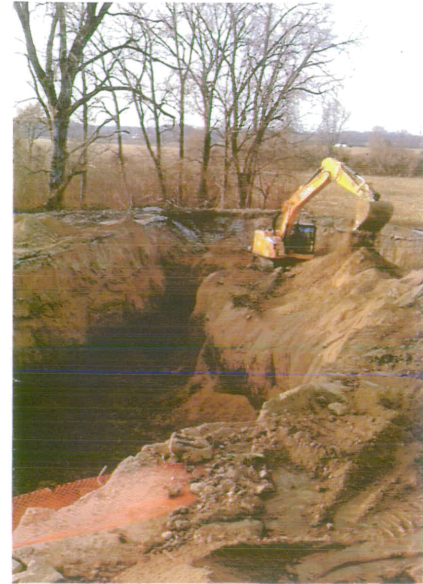
12/03/2013: View of Excavation looking from the Southeast corner toward the Northwest corner of the Excavation
